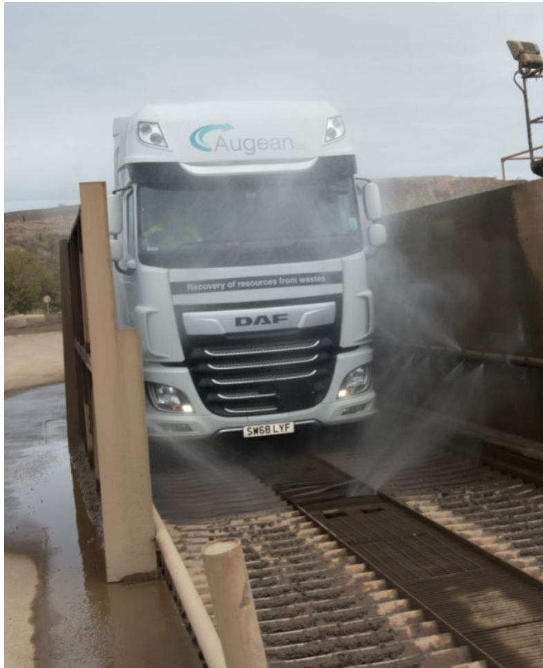
Photograph NTS 2: Wheel and vehicle body washing facilities at ENRMF
